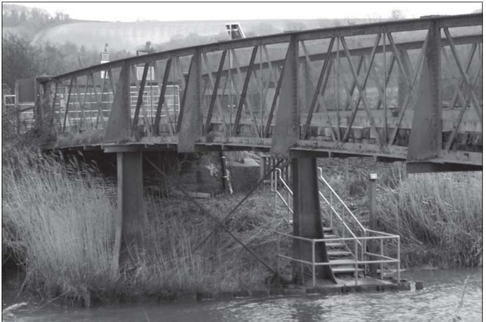
Fig 2 Close up of the pier on the east bank and the upstream truss. The level crossing over the Mid Sussex line can be seen in the background. (Chris Bryan)
