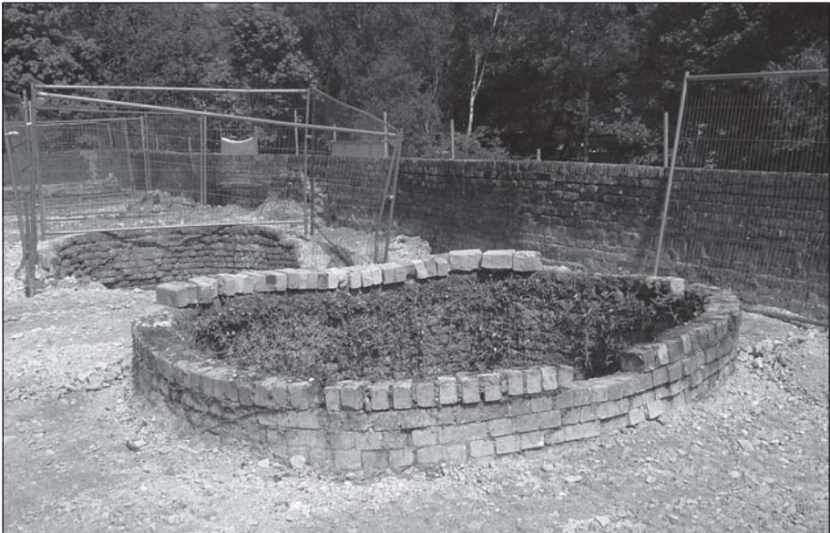
View of the top of the De Witt Kilns, prior to start of restoration.
